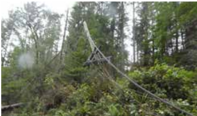
Example of infrastructure damage on Gabriola Island.
